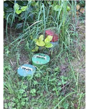
Typical Property Line Shutoff and Meter
