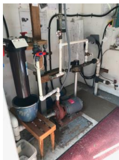
Inside Pump House
