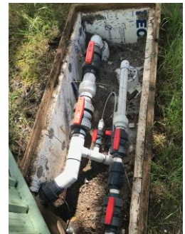
Header Tank Manifold
