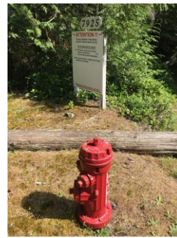
Fire Water Connection
