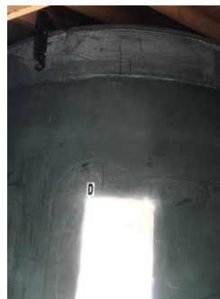
Header Tank "D"
