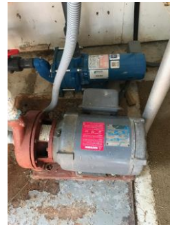
Operating and Standby Pumps
