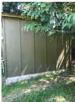
Well #2 Pump House
